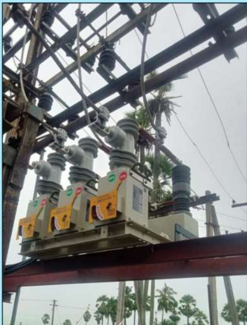
APCPDCL, Vijayawada 3-Phase to 1-Phase
